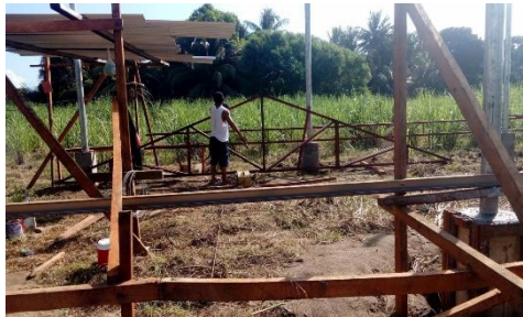
Commercial Electric Rice Mill (2) and Rice Mill House with a total amount of Php 1,000,000.00 for Polo Plantation Agrarian Reform Beneficiaries Cooperative Block Farm, Tanjay City, Negros Oriental.
