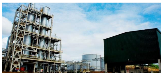
Green Future Innovations, Inc. (GFII) Bioethanol and cogeneration plant in San Mariano, Isabela Ecofuel Agro-Industrial Ecozone.
